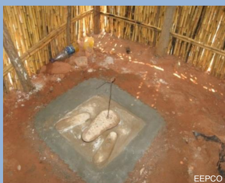
Improved pit latrine (slab is washable)
