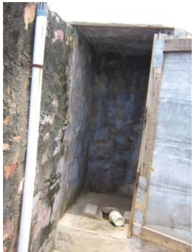
Individual Household Latrine in Mewat
