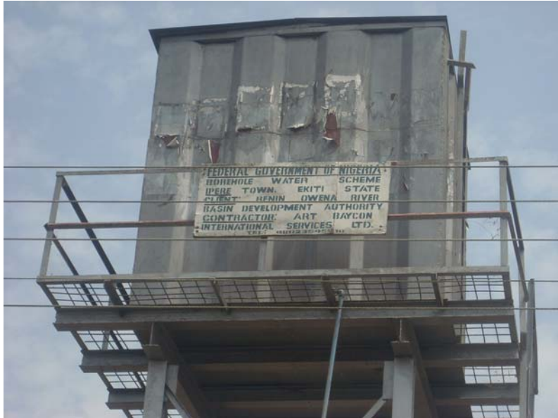
An abandoned water project in Ilejemeje LGA of Ekiti State
