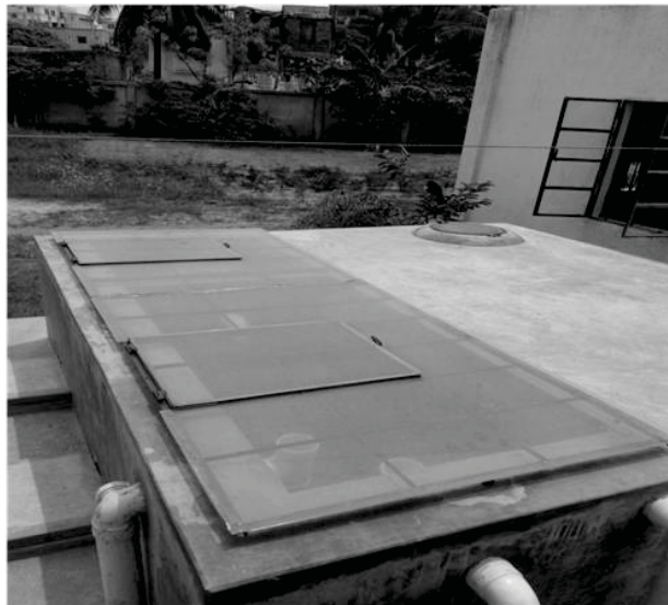
Figure 19: A sedimentation-filtration system (with rainwater storage tank) installed above ground at UITS, Dhaka.
