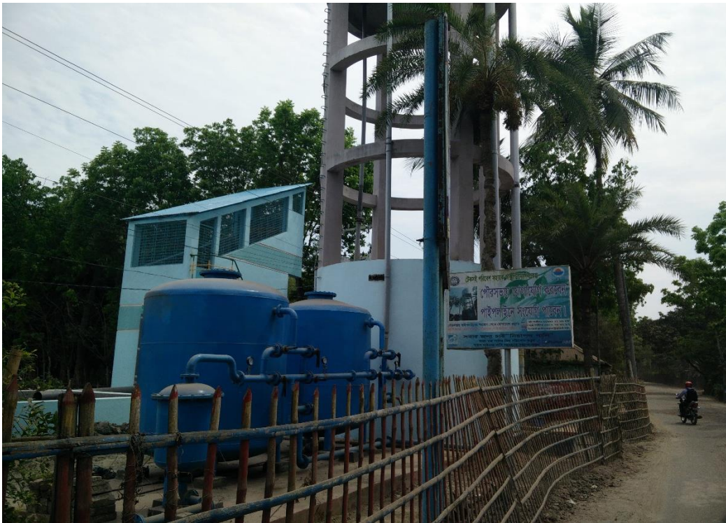
Picture 6: Water treatment plant at Paikgacha
