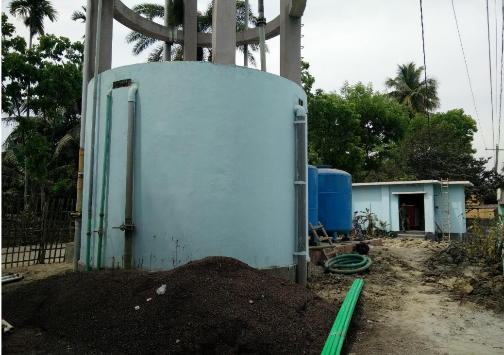
Picture 7: Water treatment plant at Paikgacha
