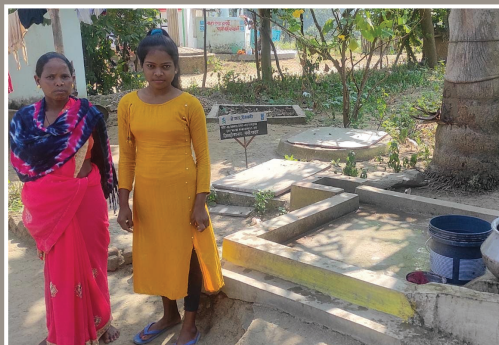
Complete unit- Leach Pit with Washing Platform and Silt chamber
