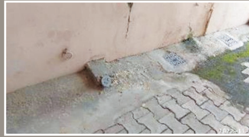
Chambers of individual houses connecting to the Community Magic Pit
