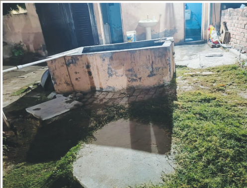
Leach pits in Bhasada in 2022- Functioning well
