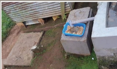
Washing platform, Grease trap with bio-filter and covered soak pit
