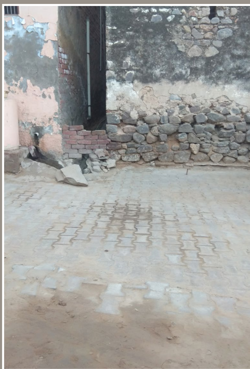
Community leach pit under the paved road-literally invisible
