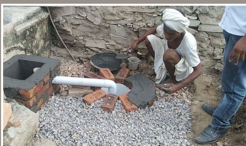
Pipe connection from chamber to pit
