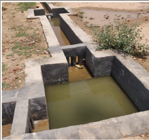
Main incoming drain from households (measurement of flow is crucial)
