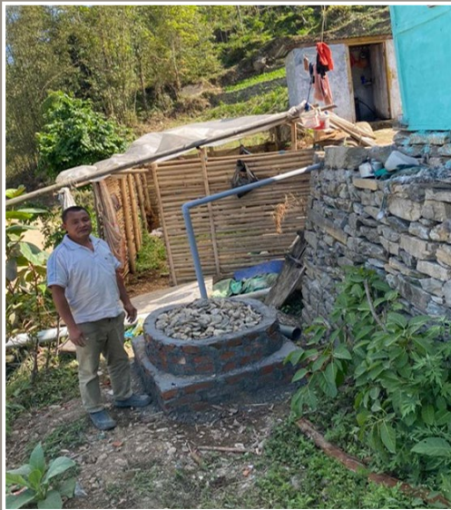
Soak Pit with brick lining over the ground
