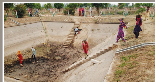
Operation & Maintenance of Facultative pond
