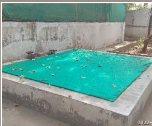
Final storage tank for treated water
