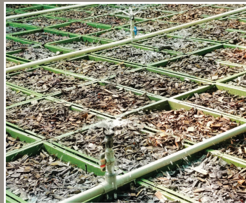
A biofilter/vermifilter unit consisting of crates filled with wood chips filled with earthworms. Effluent is sprinkled through sprinklers
