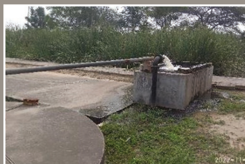
Grey water from the collection tank is pumped into the screening chamber
