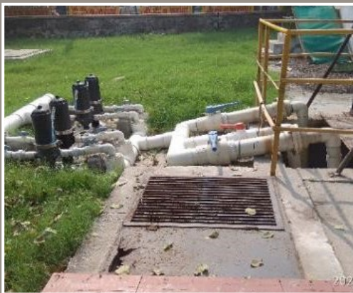
Primary Bar Screen chamber, storage tank and pumps
