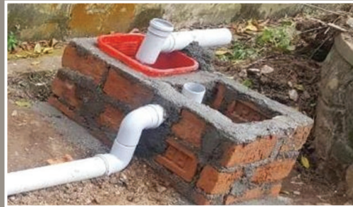
Improved grease trap cum silt chamber
