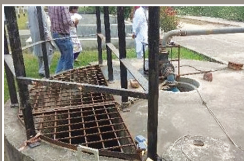
Primary Collection tank for grey water
