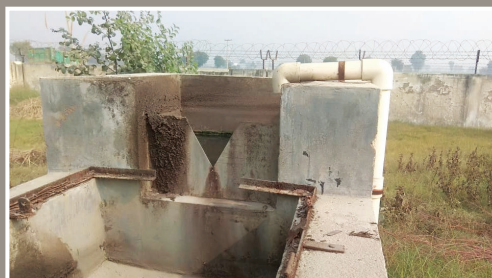
Wastewater is pumped into the planted bed
