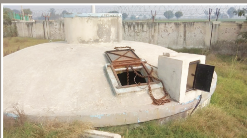
Central collection tank for wastewater
