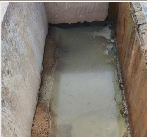
Settling tank no.3 with sand and charcoal powder
