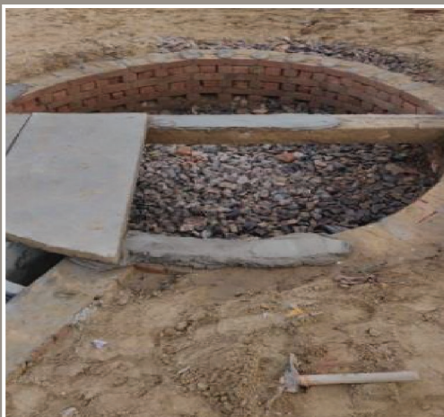
Leach pit with a honeycombed partition wall. One part is filled with brickbat/boulders
