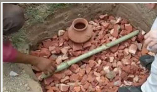
Placing the earthen pot filter over the last layer of filling medium
