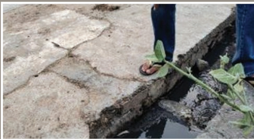
Open drains collecting liquid waste
