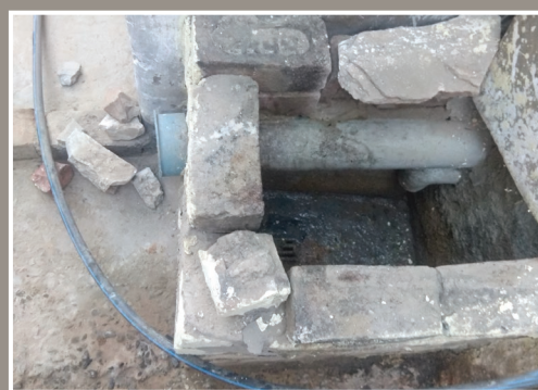
Junction chambers from individual households joining directly to the Leach Pit
