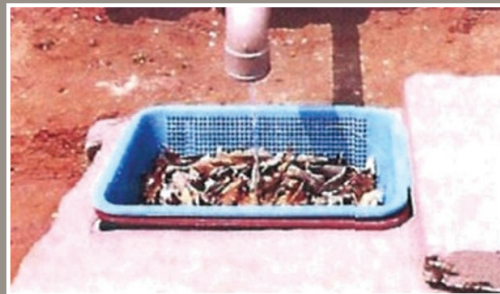
Bio-filter introduced in the plastic strainer to reduce the cleaning frequency
