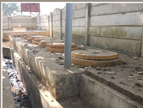
Internal View of DEWATS system showing Screen chamber, Anaerobic baffled reactors and Soak pit (at the far end)
