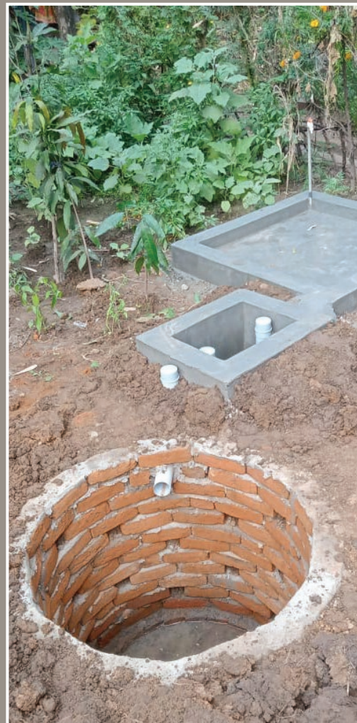
Complete unit – Washing platform, silt chamber and the leach pit
