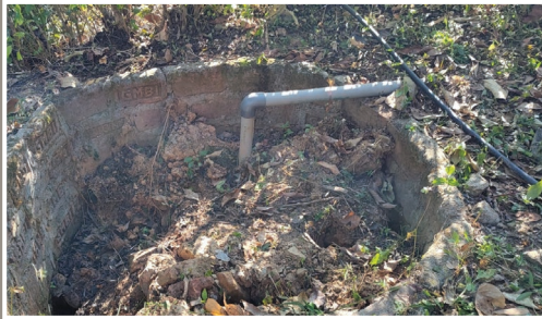
Drain pipe directly inserted in the filling medium. Pit open to the atmosphere
