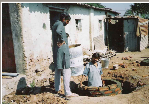
Household Leach Pit constructed in 2005
