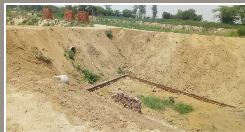
Operation & Maintenance of Anaerobic pond
