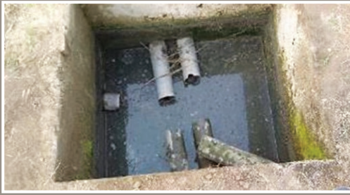
Placing a PVC drum with a row of 1.5 inch diameter holes, 10 inches from the top
