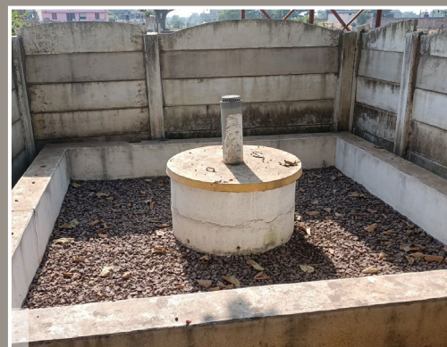
Soak Pit for groundwater recharge by the treated water
