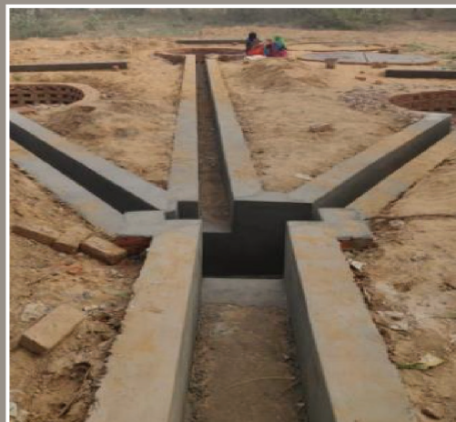
No. of leach pit ranges from 2 to 6 as per the quantity of grey water to be treated
