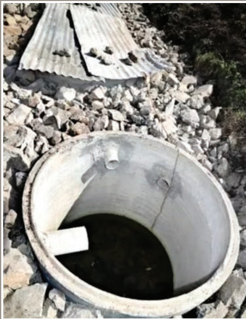
Chamber at the end of the drain
