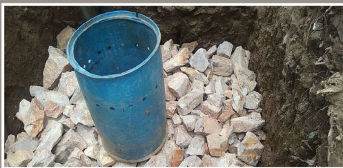
Placing a PVC drum with a row of 1.5-inch dia. holes, 10 inches from the top
