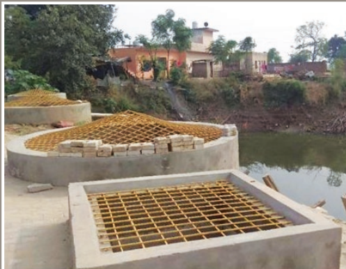
Screening chamber (square) and Filtration wells (cylindrical) in series
