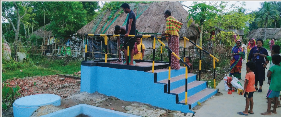
Raised washing platform, Soak Pit and a Reed Bed
