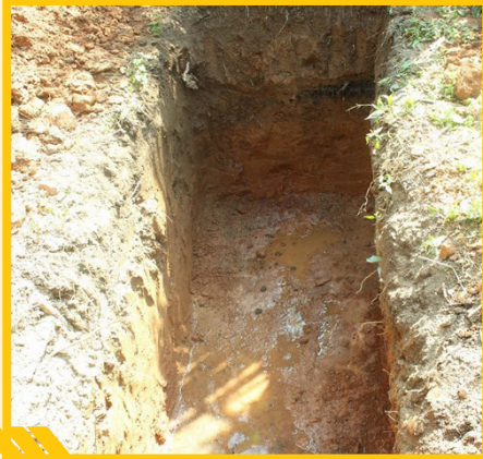
A PIT IS DUG WITH A LENGTH OF 8 FEET, DEPTH OF 4.5 FEET AND WIDTH OF 3 FEET
