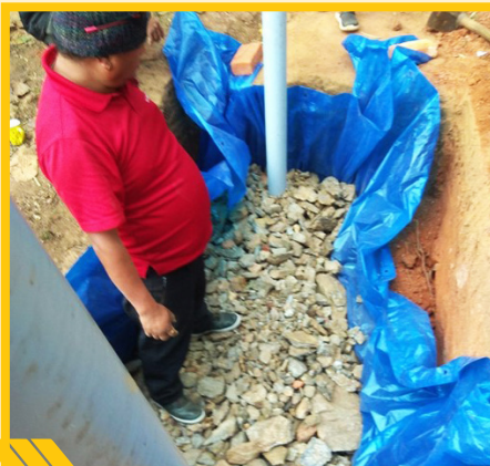
FITTING OF INLET AND VENT PIPES AND FILLING UP OF BIG STONE GRAVELS
