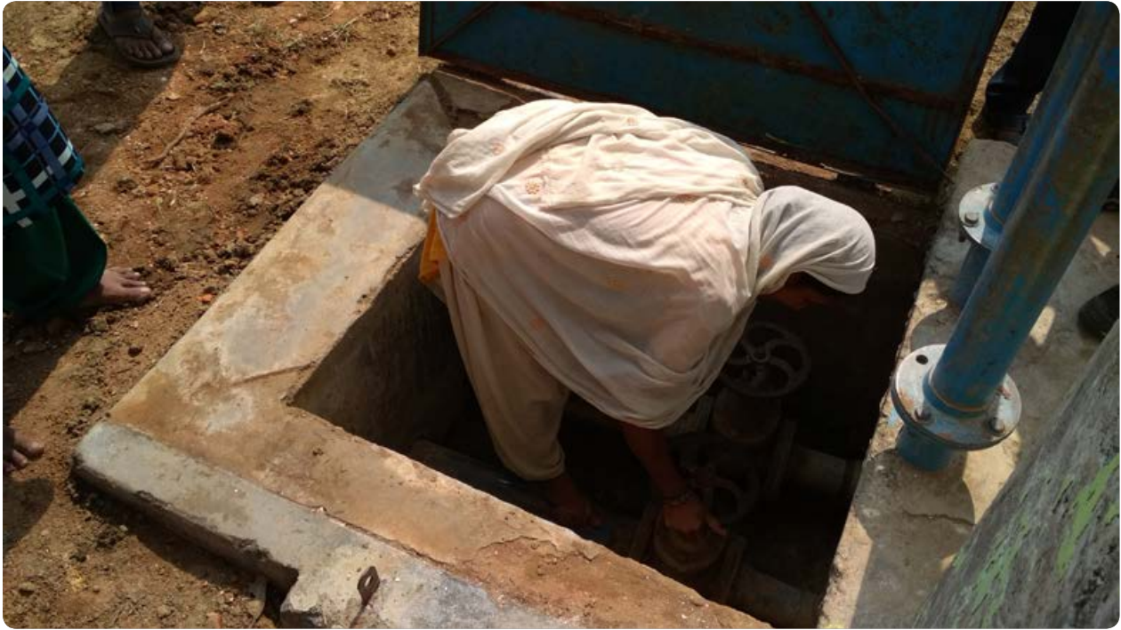
The valve of the water distribution system being opened by Zulaikha Khatun, the former operator
