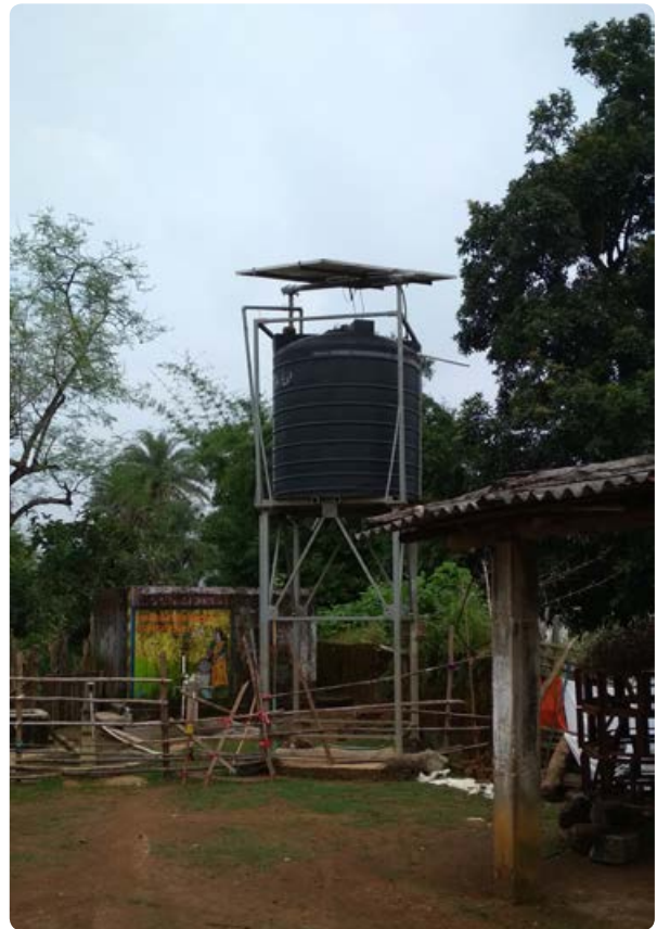
The solar-based water pumping scheme at Goyenda
